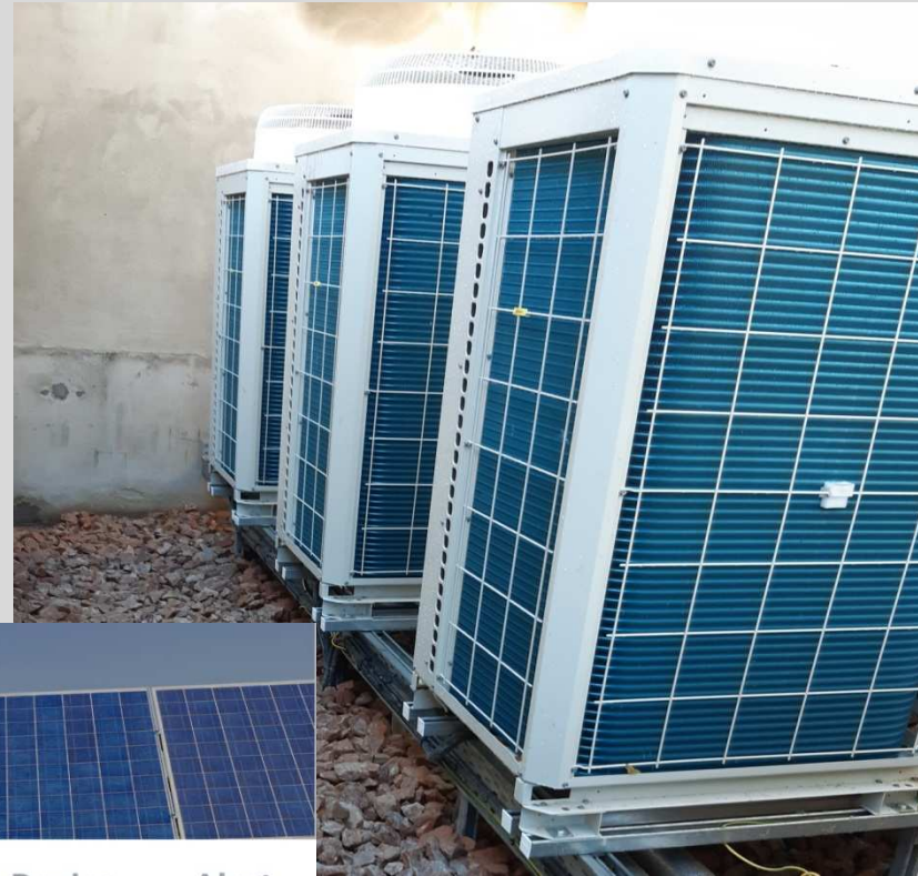
Air Source Heat Pumps
