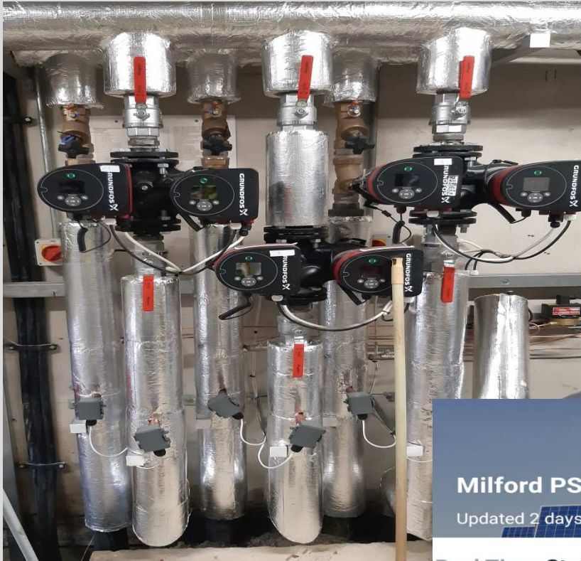
Pump Controls to BMS
